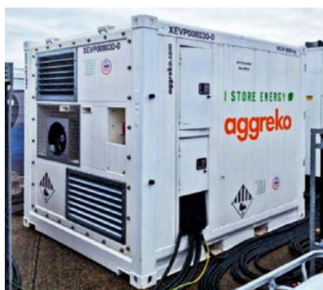
FIGURE 14: Example of a battery bank used to charge electric vehicles in Berlin. The battery bank charges slowly from the grid, but discharges quickly into the vehicles.
